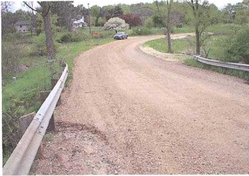
AB AVENUE LOOKING WEST AT SOUTH CROSSING PRIOR TO BMP CONSTRUCTION, JULY 2003
